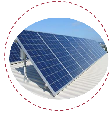
Roof top solar
